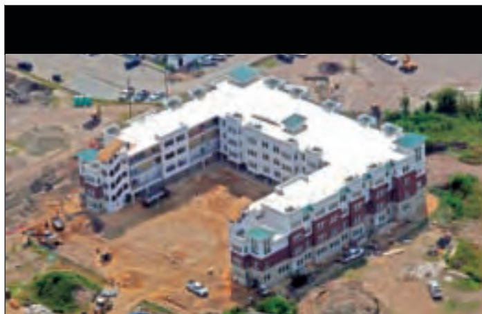
The Landmark Group has selected McShane Construction's Auburn office to complete the new 60-unit West Yard Lofts affordable housing development located at the former Charleston Naval Base in North Charleston, South Carolina.
